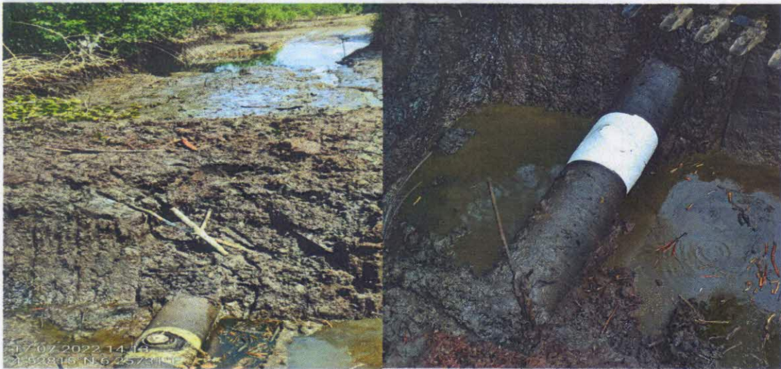
PICTURE 1: SHOWING THE INCIDENT POINT AT 12 O' CLOCK POSITION OF THE PIPELINE.
